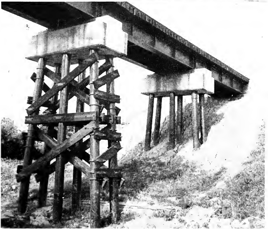
Fig. 1 (above)—General view of bridge and test train at Fillmore, Ill. Fig. 2 (below)—View of pier 3, showing type of timber bracing used.
